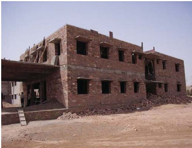
Building a hospital for poor people of a rural area in the Thar Desert (Jodhpur, Rajasthan, northwest of India): a project financed by the Japanese government's grassroots human security grant aid.
