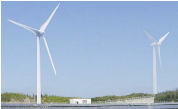
A demonstration plant for solar power generation (490 kW) and two wind power generators (900 kW each, to be completed in September 2007)
