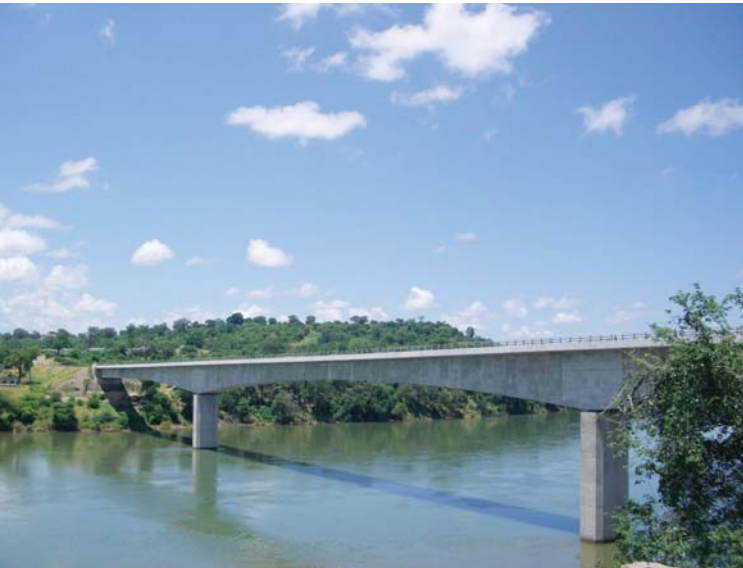
Chirundu Bridge: Completed on Oct. 31, 2002, with Japan's grant aid, this bridge is part of the Beira Corridor, an international highway between Zimbabwe's capital Harare and Zambia's capital Lusaka. It has contributed in the improvement of local transportation.
