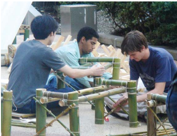
Students from Japan and the United States work side by side on constructing temporary street furniture they have designed for Kanda, a Tokyo district packed with antiquarian bookshops.
