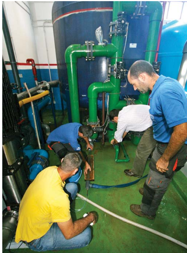
The vortex machine attached to reverse osmosis reducing energy by 70%
