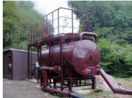
Power generation using heat from a hot spring at Tsuchiyu Onsen in Fukushima
