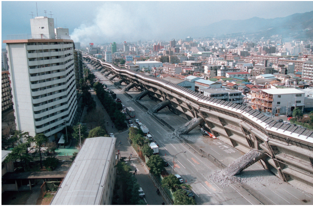
The Hanshin Expressway in Kobe's Higashinada Ward collapsed on January 17, 1995 during the Great Hanshin Earthquake, which struck at 5:46 a.m. that day. The 7.3 magnitude quake that hit the city of Kobe and nearby areas in Hyogo Prefecture left 6,434 people dead and 43,792 injured.
