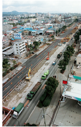
The collapsed expressway near Fukaebonmachi in Kobe's Higashinada Ward was completely cleared up within a month of the earthquake.
