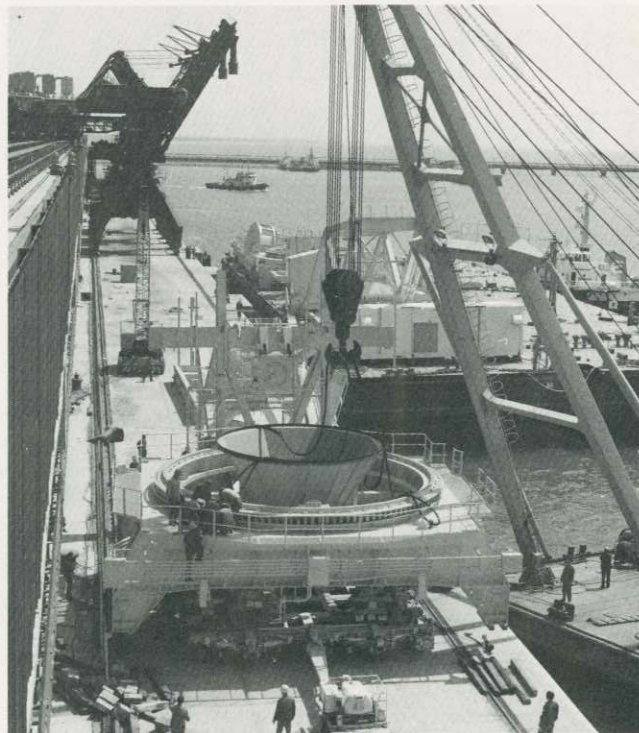
Coal wharf under construction at Qinhuangdao. This is one of China's key projects under the sixth five-year plan.
