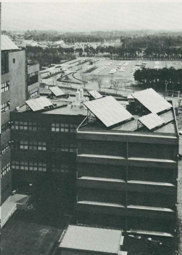
Photovoltaic power generation system at Tsukuba University in Ibaraki Pref.
