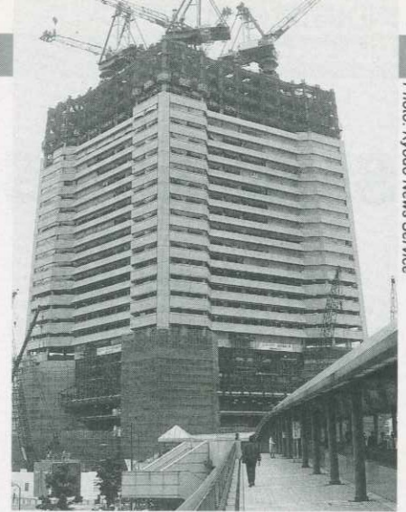
An increase in projects for high-rise buildings has spurred demand for large cranes.
