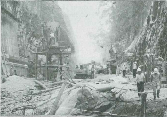
Economic cooperation in the Asian region desires a shift from public to private hands—dam construction site in Indonesia.
