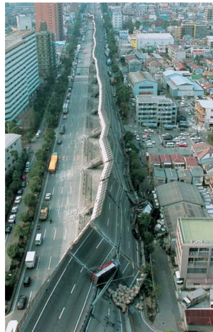
The pillars supporting this expressway in Kobe collapsed during the Great Hanshin earthquake
